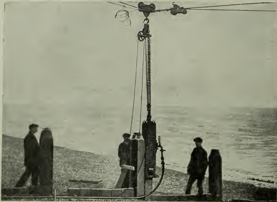
A No. 5 Hammer driving timber piles at Hythe, suspended from a cable.
